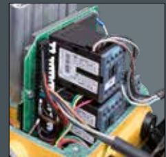
LOW VOLTAGE CONTROL
